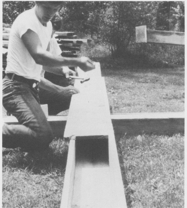
A beaver pipe allows water to pass underneath a beaver dam, preventing the flooding of nearby roads and controlling the water level. This beaver pipe was constructed and installed at Surry Mountain Lake Dam in Surry, New Hampshire.
