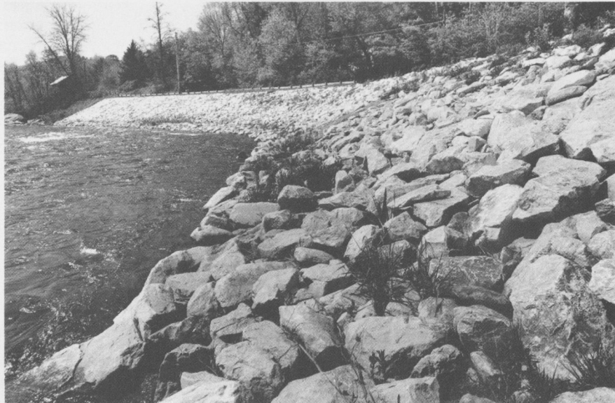
Stone slope protection, a layer of large stones usually underlain by a layer of gravel bedding, reduces erosion from streamflow and waves. The stone slope protection on the Housatonic River in Salisbury, Connecticut, strengthens a 350-foot reach of the riverbank and stabilizes the roadway.
