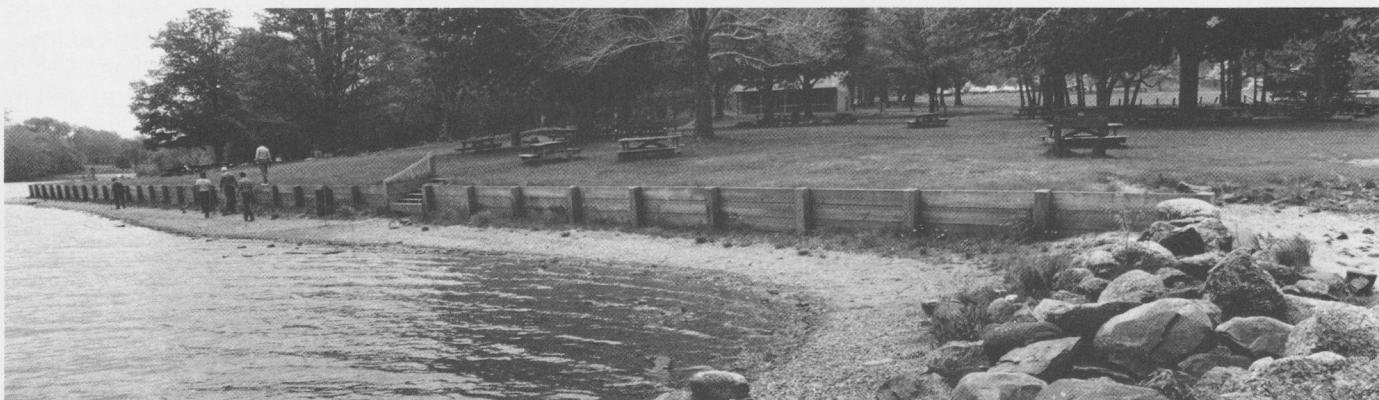
The timber bulkhead at Squantz Pond State Park in New Fairfield, Connecticut, prevents sliding of the land and protects the bank from erosion.
