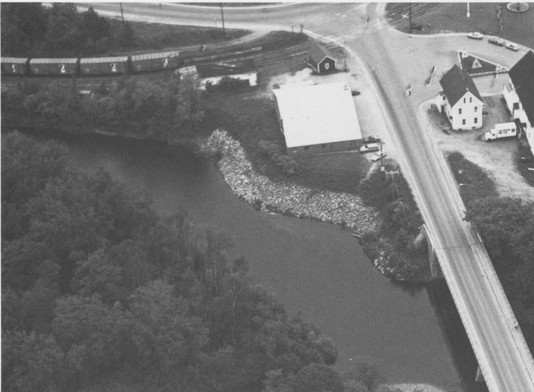
About 300 feet of stone slope protection along the Connecticut River in North Stratford protect a fire station that had been threatened by erosion.
